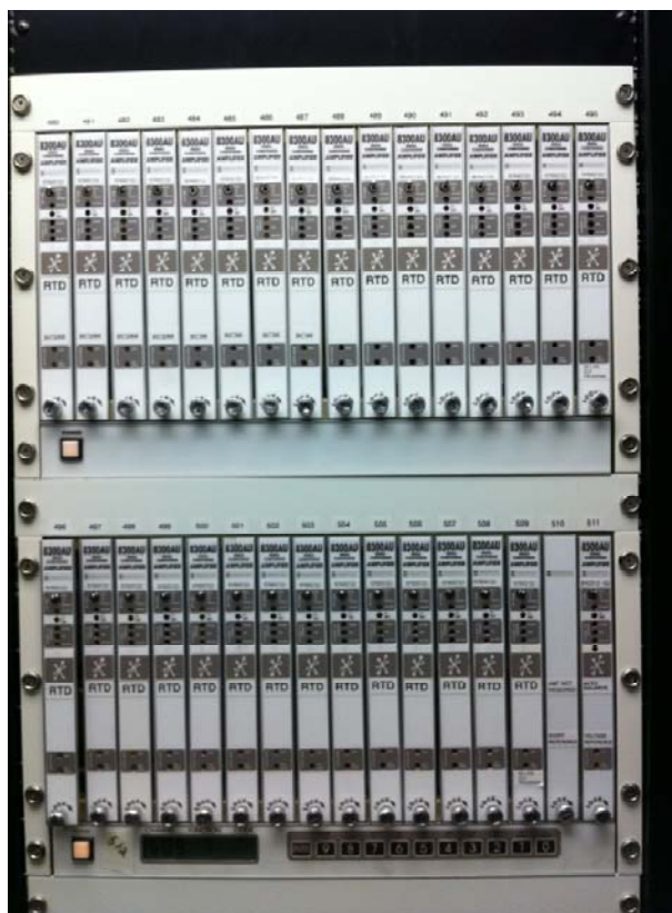
Figure 9, Preston 8300AU Signal Conditioners
