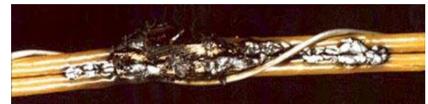
Example of arc tracking
