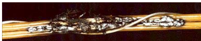
Figure 30: Example of arc tracking
