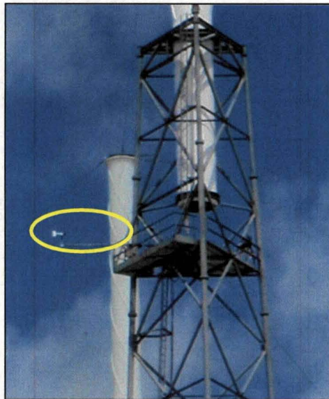
Figure 18. The SLC 41 southeast lightning protection tower and wind sensor, looking west-northwest. The sensor and boom are highlighted by the yellow ellipse. The top of the southwest lightning tower is in the background.
