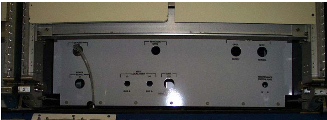
Figure 8. CHeCS Rack: Utility Interface Panel
