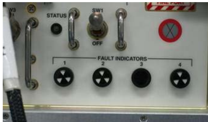
Figure 54. Example Fault Indication after an automatic shutdown
