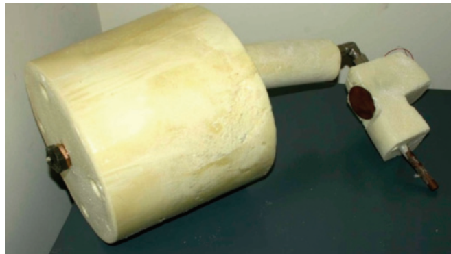
Figure 63. Insulated LN 2 accumulator and condenser.
