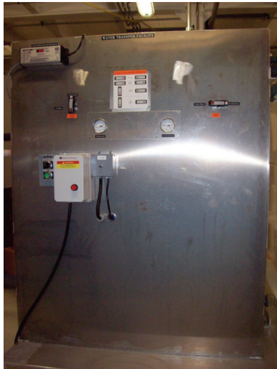
Figure 75. Water supply system control panel.
