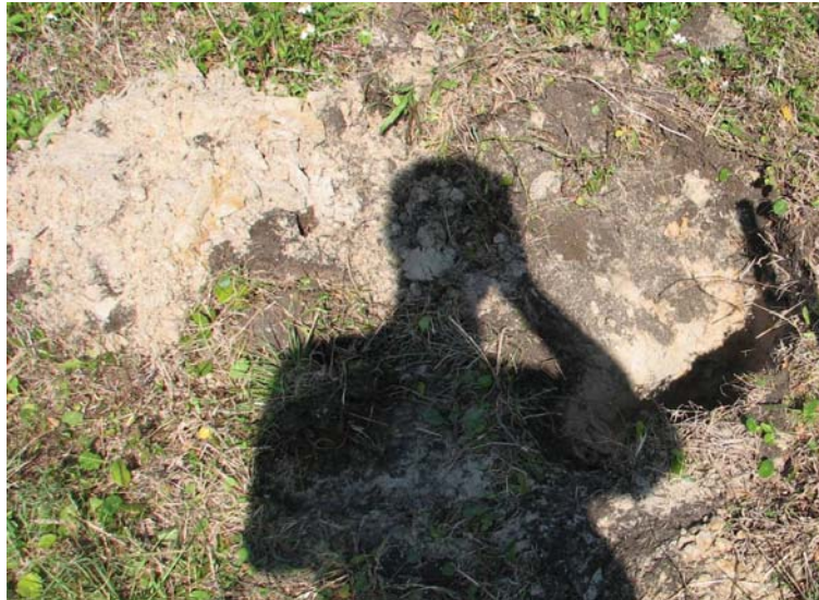
Figure 5-1: Excavation at Pad 39 B, inside ring road. Topsoil is brown. Underlying sand is tan.
