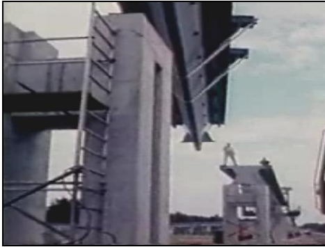
MAGLEV Pylons and Rail Segments
