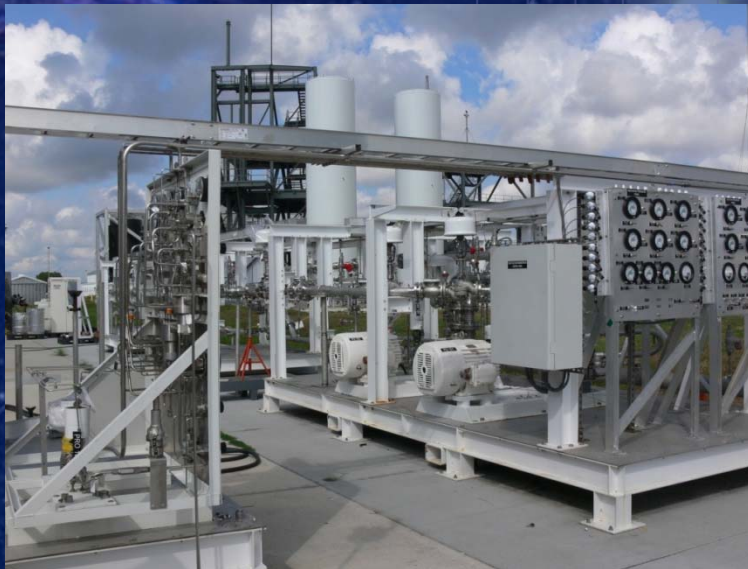
Pump and Control Skids
