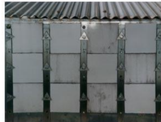
Exposed outside for 1 year
