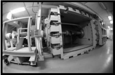
M6 Nozzle Test Chamber (B1247D) Idle, requires refurbishment
