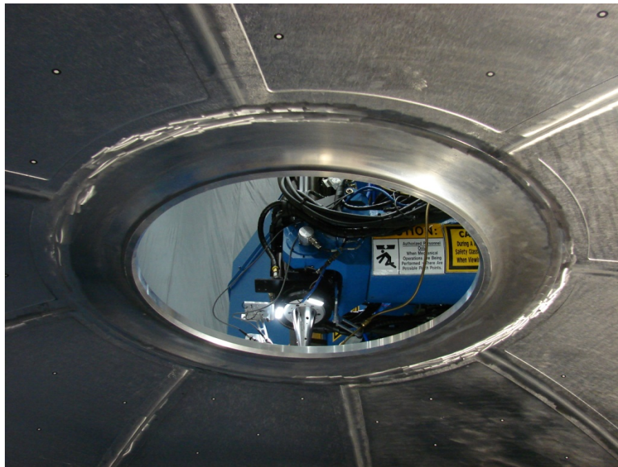
Figure 7 - Welded Manhole Fitting
