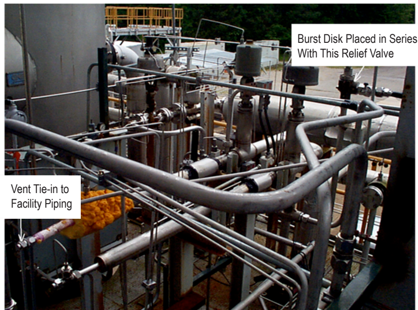
Figure 10. Facility LH 2 vent tie-in to back-pressure control.
