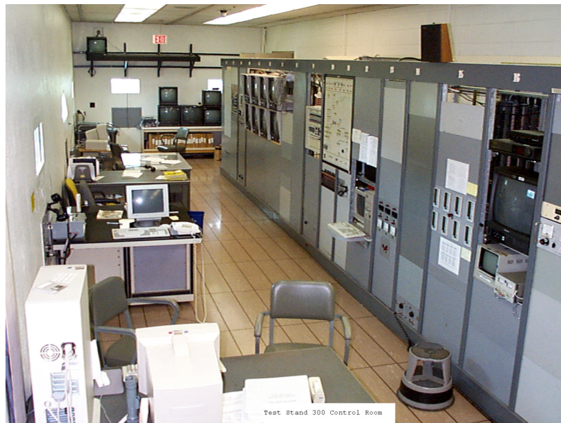
Figure 12. Control room for TS300 vacuum chamber.
