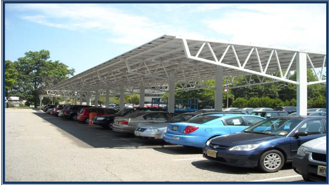
Figure 7. Typical Solar panel installation for parking areas. (Photo Courtesy of Andrew T. Nekus P.E., SunDurance Energy, anekus@SunDuranceEnergy.com, www.SunDuranceEnergy.com, A Conti Group Company)
