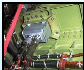
Aft Compartment Hydrogen Monitoring
