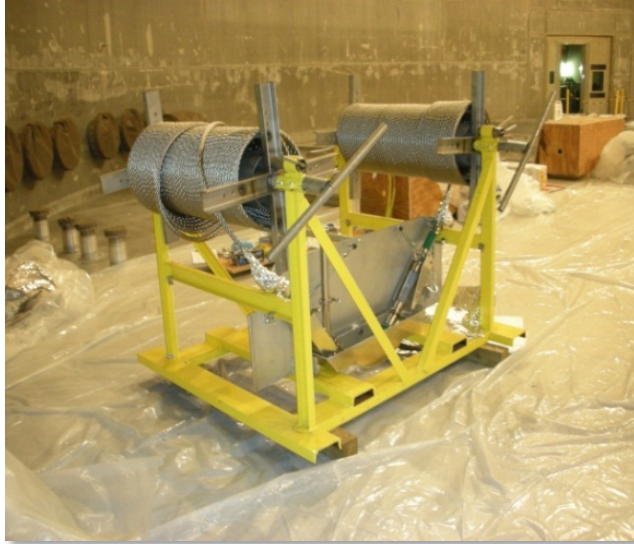
Figure 10.—Arrangement for applying low vapor pressure oil to hoist wire ropes.
