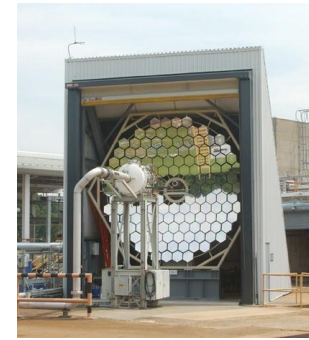
10kW solar Facility at MSFC
