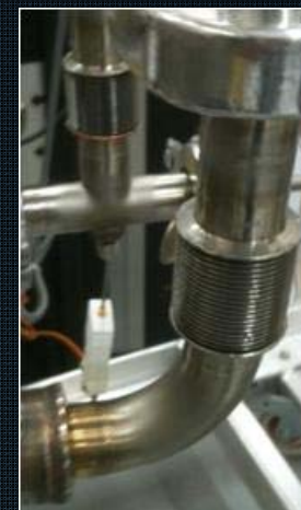
H 2 and Ar Reactor Inlet Bellows
