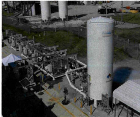
Overall view of the Simulated Propellant Loading System located at the CryoTestLab
