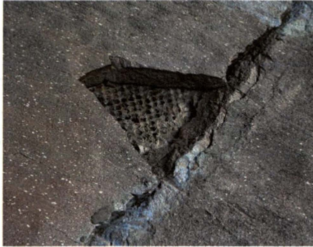
Figure 6. STS-126 Spalled and Dislodged Concrete Section
