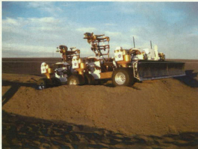
Figure 11 - Chariot Mobility Platform using the LANCE Blade to Build a Berm in Moses Lake, WA.
