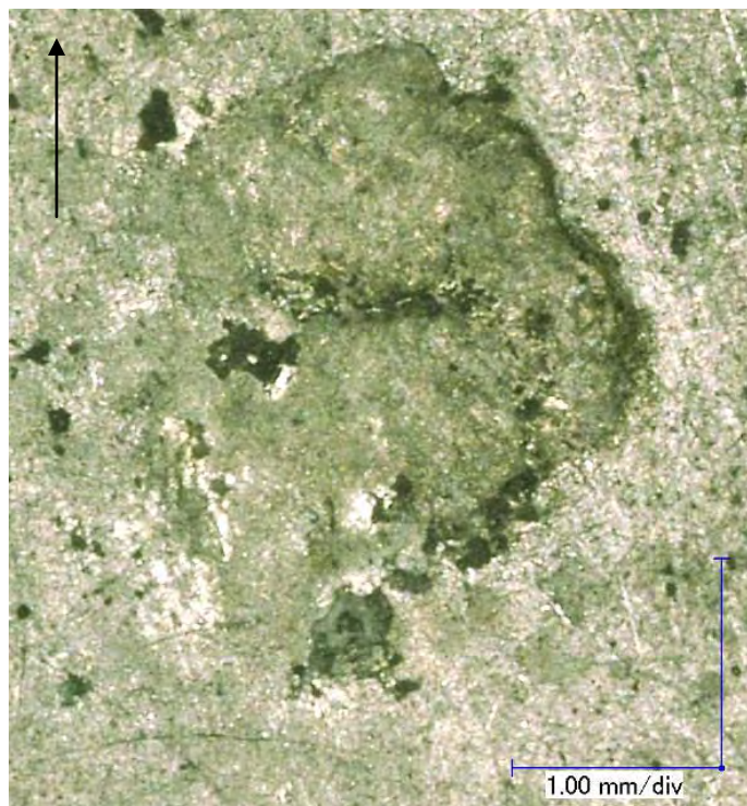
Figure 483 Close-up View of Most Significant Damage to Front of Rear Wall (black arrow indicates flight path of projectile / damage within red circle in Figure 482)
