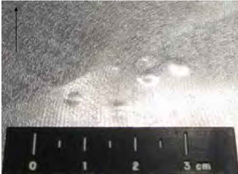
Figure 406 Close-up Oblique Side View of Damage on Back Side of Rear Wall (scale in 5mm increments / black arrow indicates flight path of projectile)
