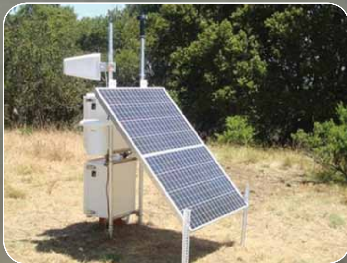
Left: One of QuakeFinder’s sensor installations. Background: The San Andreas Fault.
