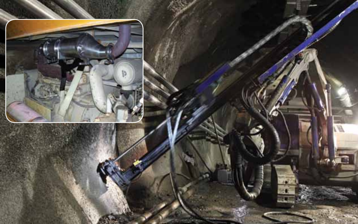
Airflow Catalyst Systems' EZ-series of converters, derived from technology developed and licensed by NASA, are used in the exhaust systems of underground diesel mining equipment to purge the air of potentially dangerous fumes. An EZ converter is installed for such an application (inset image).
