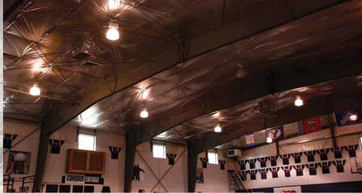
A recreational gymnasium became too hot and uncomfortable to use during the summer months, but now with RadiaSource on the rafters, the owner says the gym stays cool. The image on the background of this page shows a close-up view of the perforated material.
