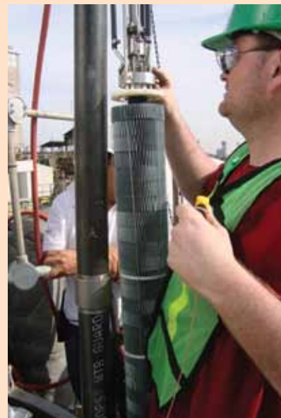
128 Reactors Save Energy, Costs for Hydrogen Production
