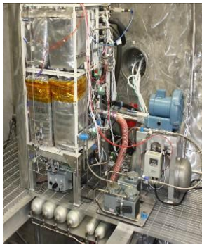
Figure 5. Carbon dioxide removal equipment. CO 2 accumulator tanks and the compressor are visible.
