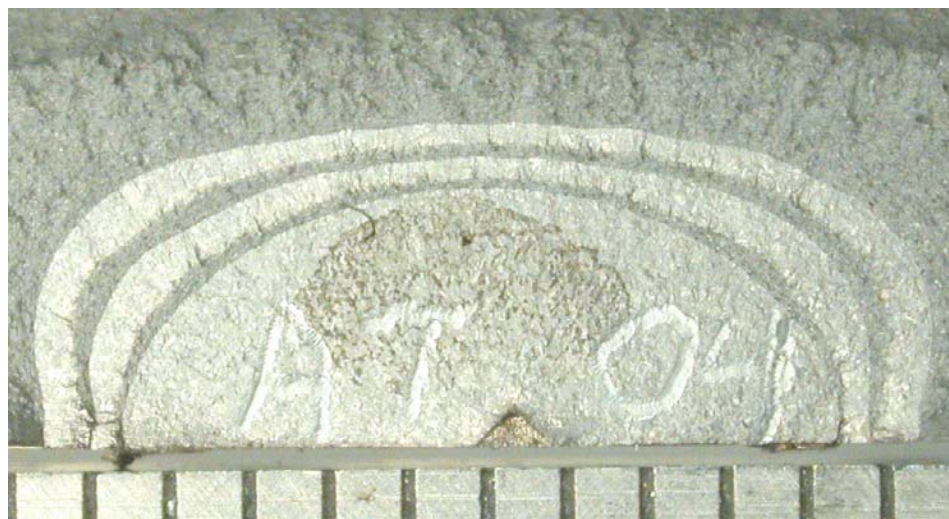
Figure 3-2.a Typical Surface Crack Fracture Surface (Tension)
