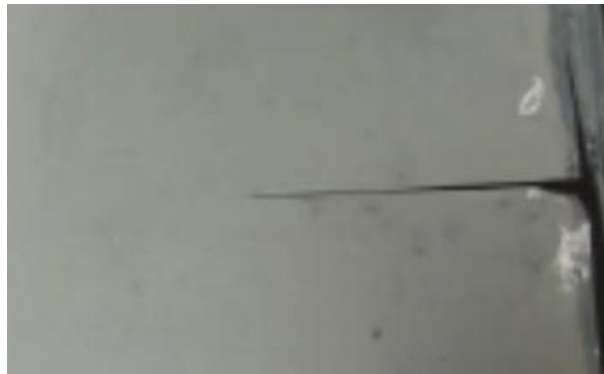
Tear on Separator
