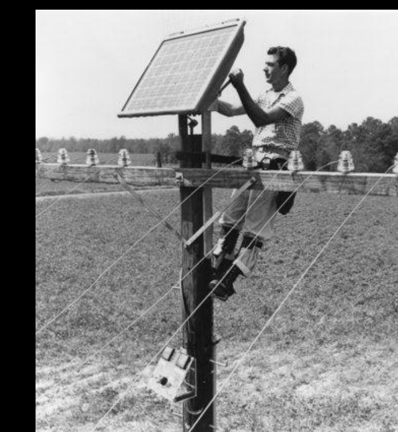
Technician from Bell Labs installing a solar PV array for a first trial. Bell Labs went on to provide solar cells for NASA.
