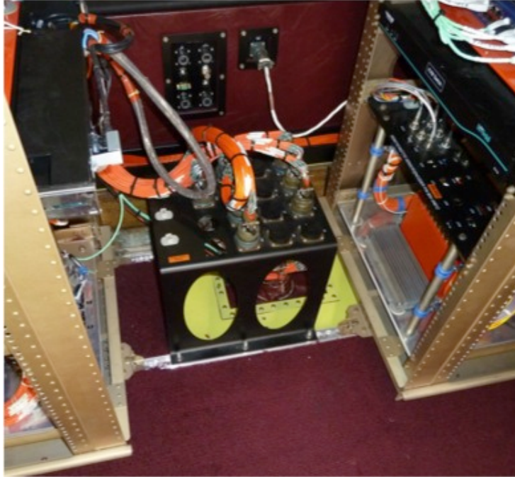
Figure 14. Sensor disconnect panel.
