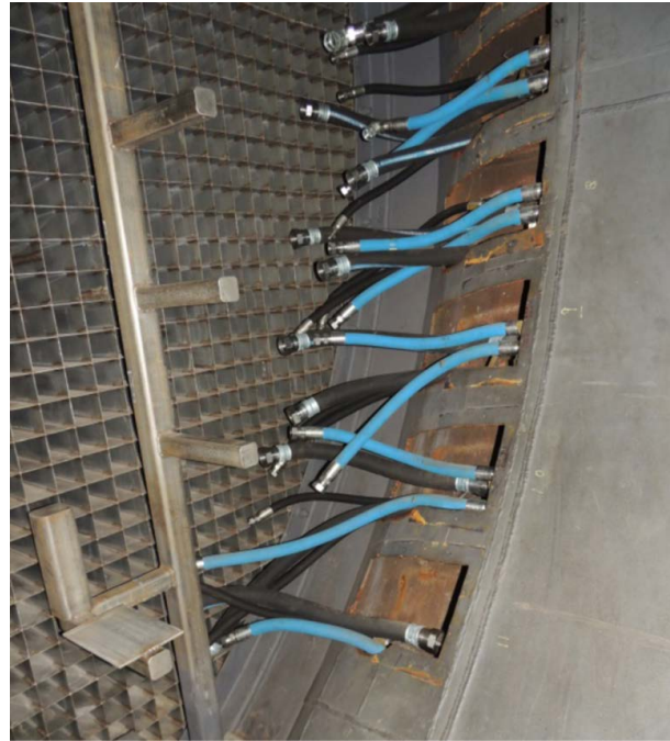
Figure 10. Supply hoses to spray bars.
