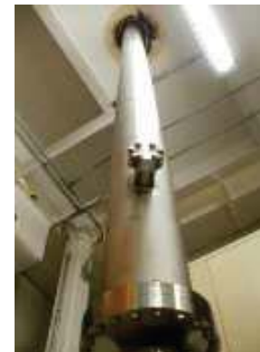
Cryogenic Container located at MSFC (below deck)
