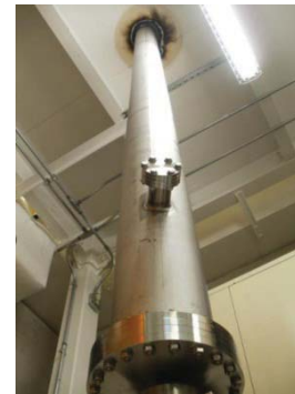
Cryogenic Container located at MSFC (below deck)
