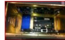
Power Control Unit (PCU)
