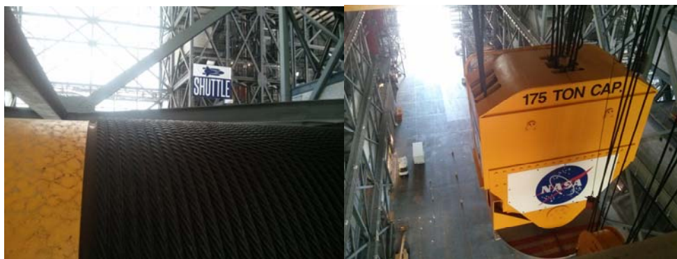
Figure 3. Properly spooled and reeved wire rope on the Vehicle Assembly Building 175-ton overhead crane. Left: Spool on drum. Right: Primary and auxiliary hook blocks with reeving. Credit: author.
