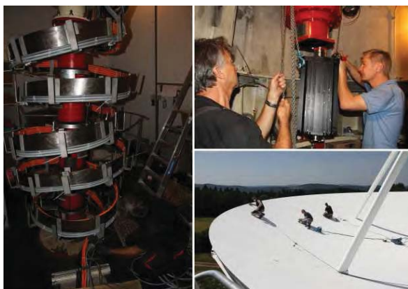
Fig. 1 Some replacement work at the RTW: new setup of the cable wrap (left), replacement of the gears and motors (upper right), and new varnishing of the reflector surface (lower right).
