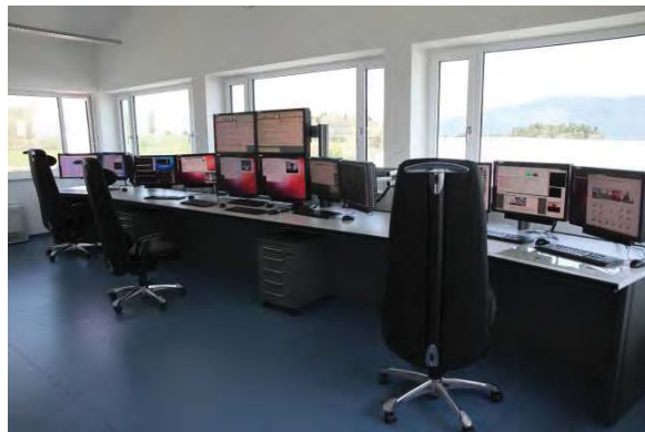
Fig. 4 The new control room and Data Center in the Twin operations building.
