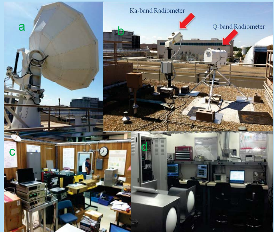
(a) 5.5 Meter Diameter Beam Waveguide Antenna on top of Bldg. 55 (b) K-band and Q-band radiometers collecting Data in roof of bldg 55; (c) & (d) RF Propagation assembly, component test, and station monitoring areas in bldg. 55
