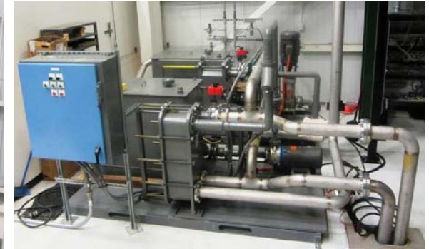
New Cooling Water System now provides 2 separate systems that cool induction coil and power feedthrough, induction heater and H 2 N 2 mixer respectively
