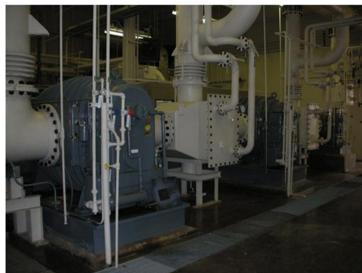
Stage-2, stage-3, and stage-4 blowers
