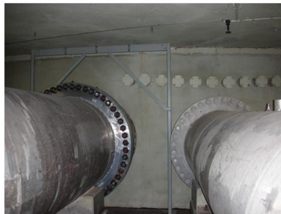
Chamber and annulus piping
