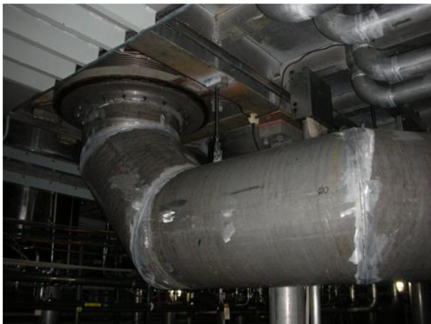
Inlet chamber piping
