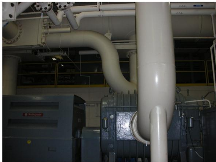
Piping at stage-1 blowers
