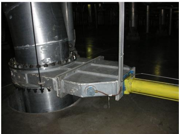
Chamber piping isolation valve
