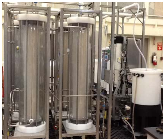
Newly assembled MABRs. The Forward Osmosis Secondary Treatment system is to the right
