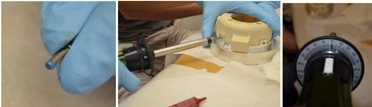
Figures 1, 2, and 3: SDP Enclosure Top getting attached to the SDP Adapter Plate.
