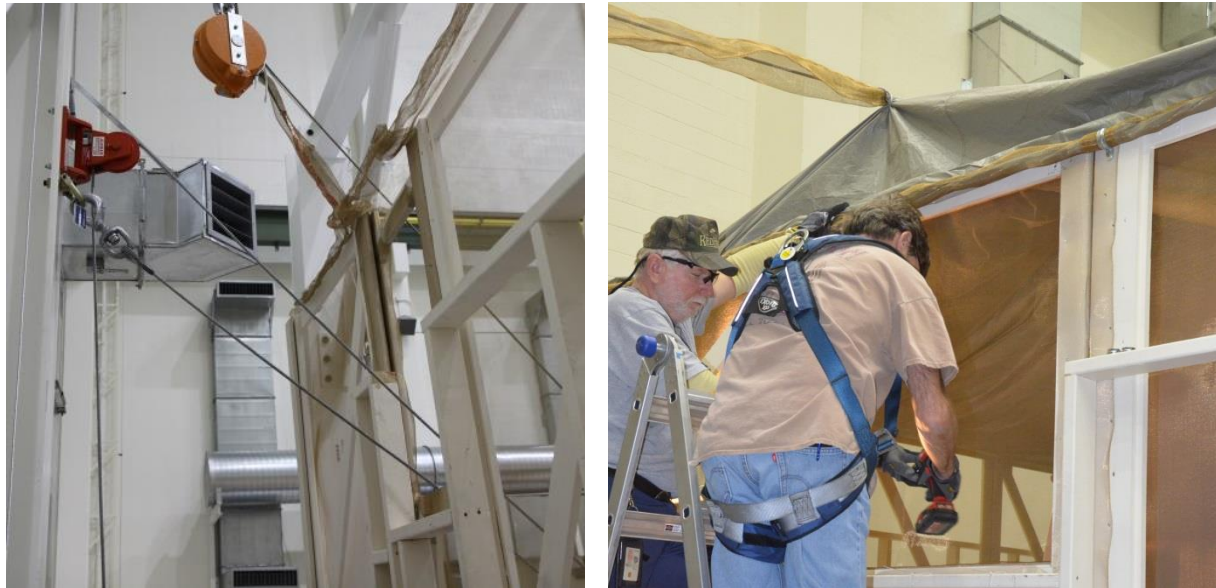
Figure 27: Flip Platform Winch Line Access (L) and Replacing the Panel Below the Safety Stay Penetration Through the RF Fabric Roof (R)
