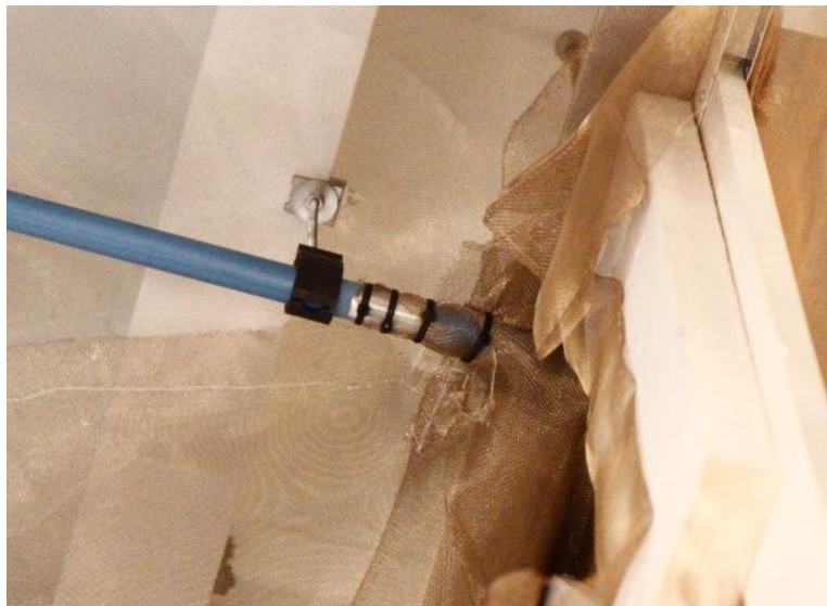
Figure 26: Socked and Mitigated Compressed Air Pipe Penetrations
