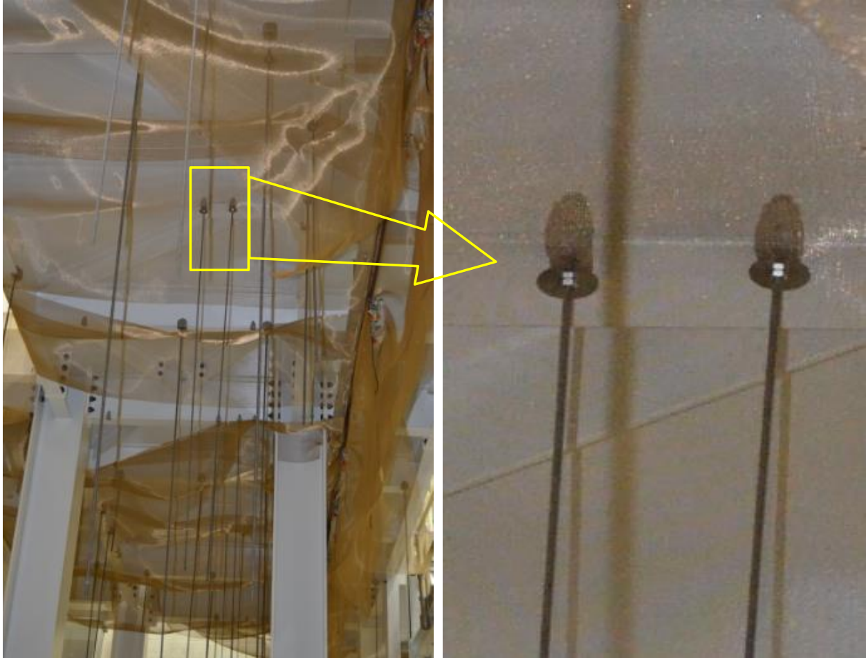
Figure 22: Threaded Rod Challenge – Close-Up of Fender Washer Installation (The two columns in the left image are those mitigated in the “C” images in Figure 21)
