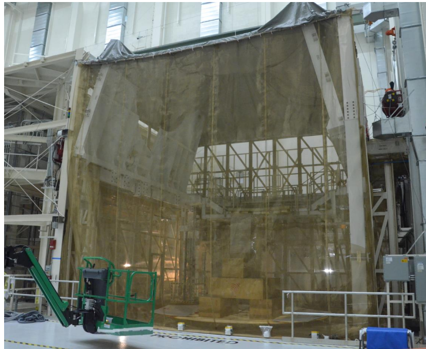
Figure 5: EMI Screen Room Ready for Effectiveness Test
