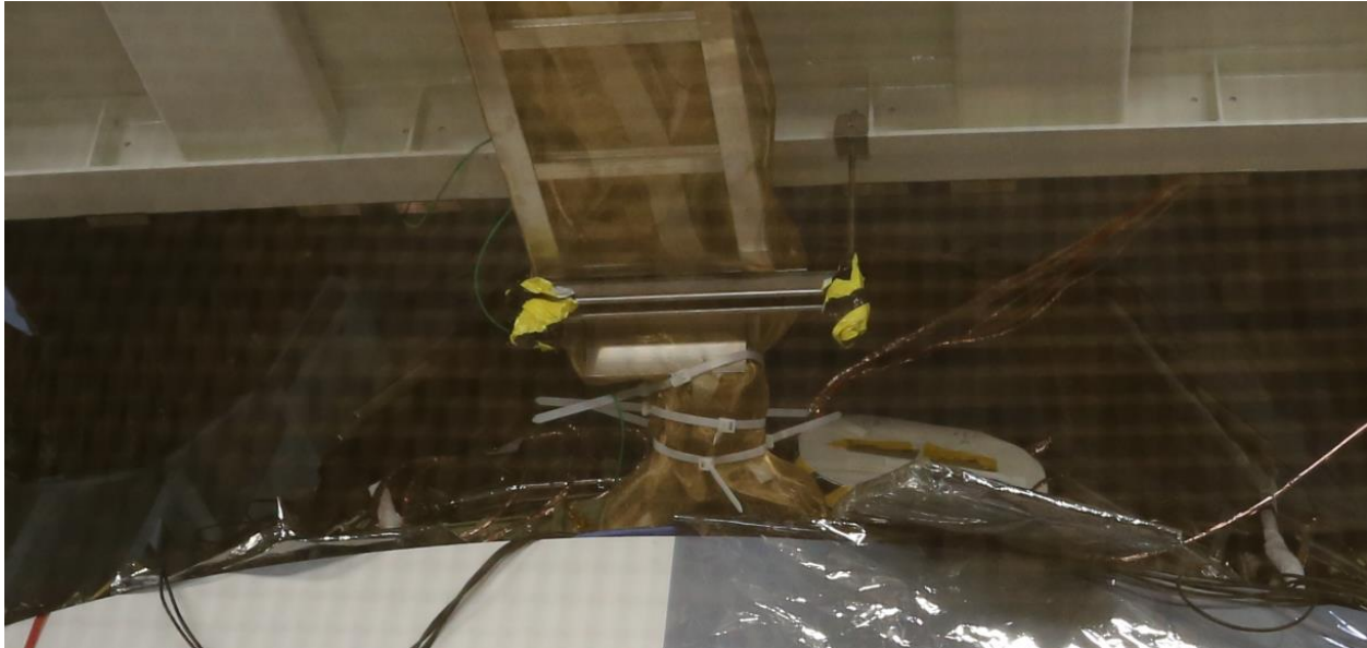
Figure 24: Socked Cables Coming Out of the Central Cable Tray
