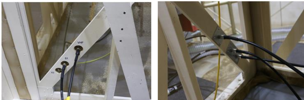
Figure 28: Antenna Horn ‘Patch Panel’ – outside (L) and inside (R)
