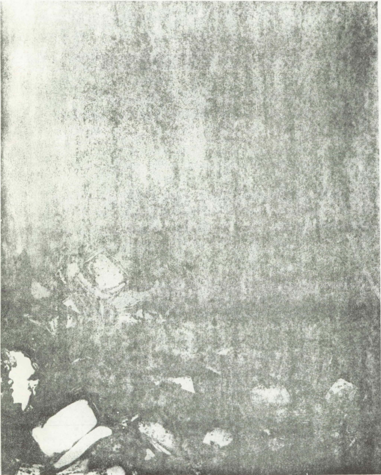
FIGURE 9. "TYPICAL" ROOM AFTER FIRE
