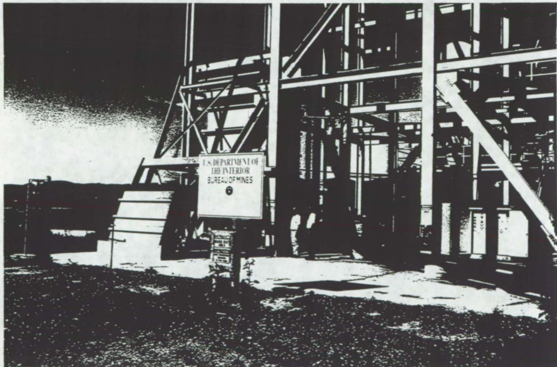
FIGURE 2b. Ground-level view of the pilot-scale ALH showing the coal skip, 30-ton-capacity coal bin, hydrohoist piping, and control panel.
