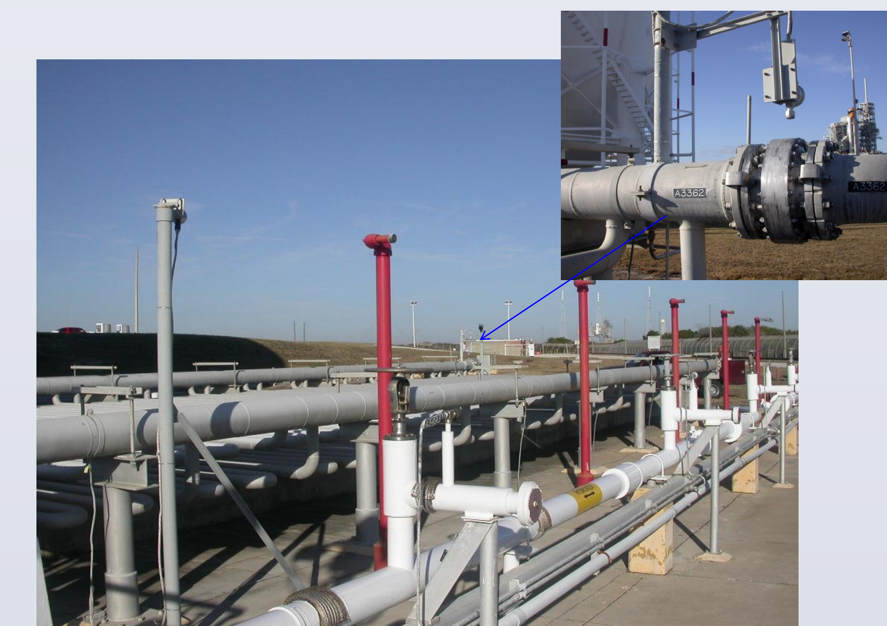
Testing on hydrogen pressurization lines during tanker loading.
