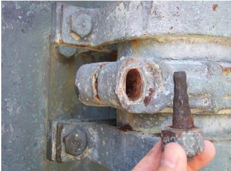
Pad 39B MLP-1: Bolt from Victaulic joint on center upper shield
