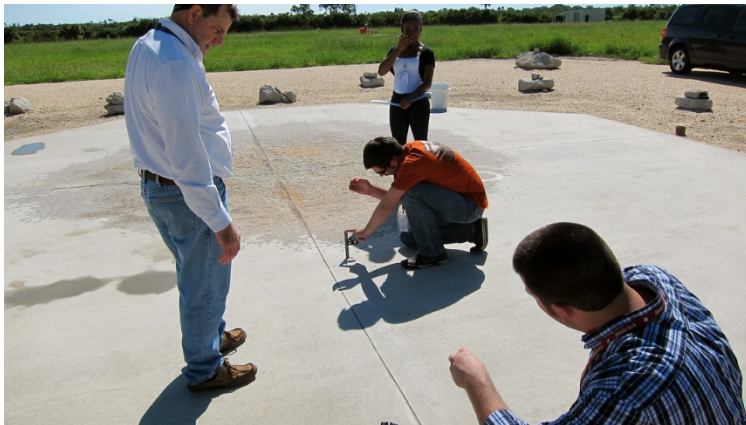
Figure 7. Determining the diameter of the eroded concrete and the erosion depth at various locations.
