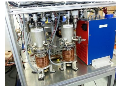
CO 2 Freezers and Chiller
