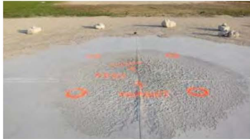
Physical state of the concrete landing pad after ten free flights.
