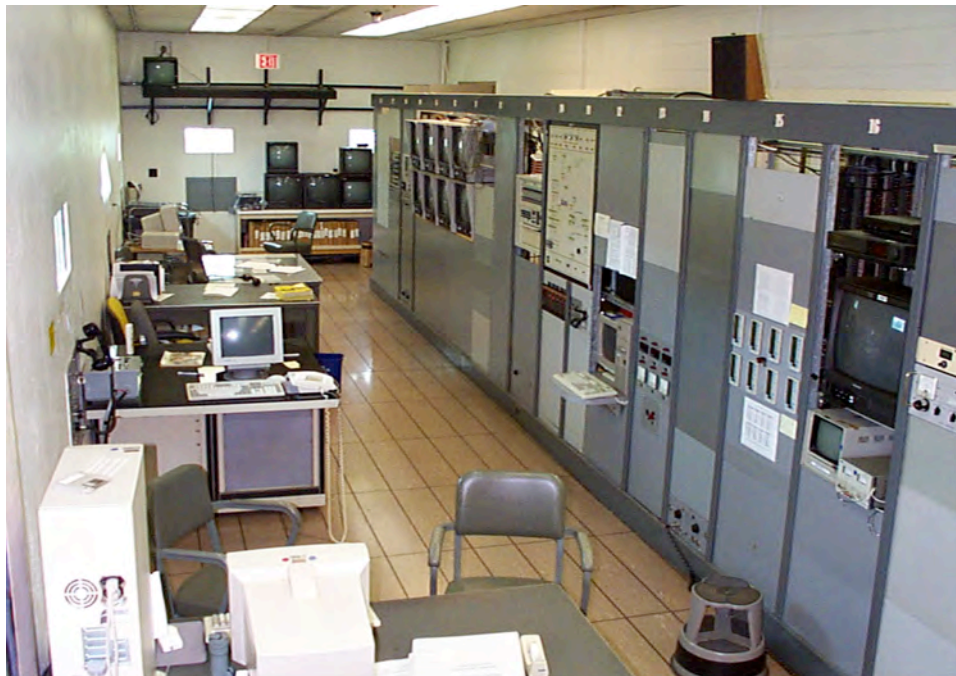
Figure 10. Control room for TS300 vacuum chamber.
