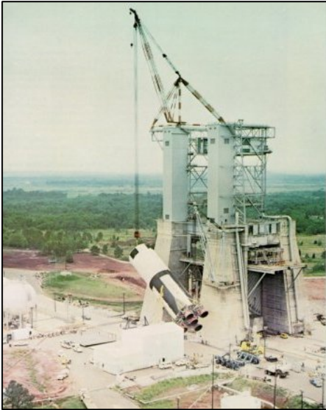
Figure 2 MSFC Saturn V Test Stand with Saturn V First Stage being lifted into place
