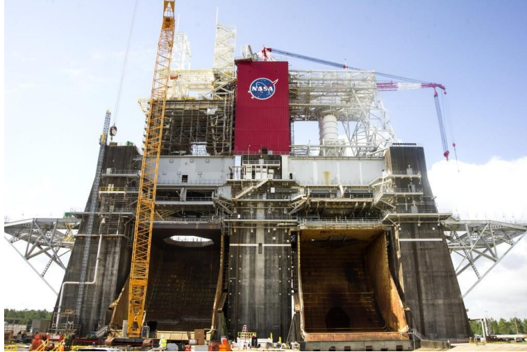
Figure. X: Structural steel for core stage testing erected on B-2 test stand at SSC site.
