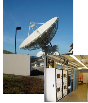
6 Ground Earth Stations
